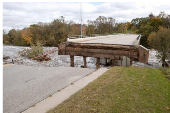
A road bridge washed-away by flooding
